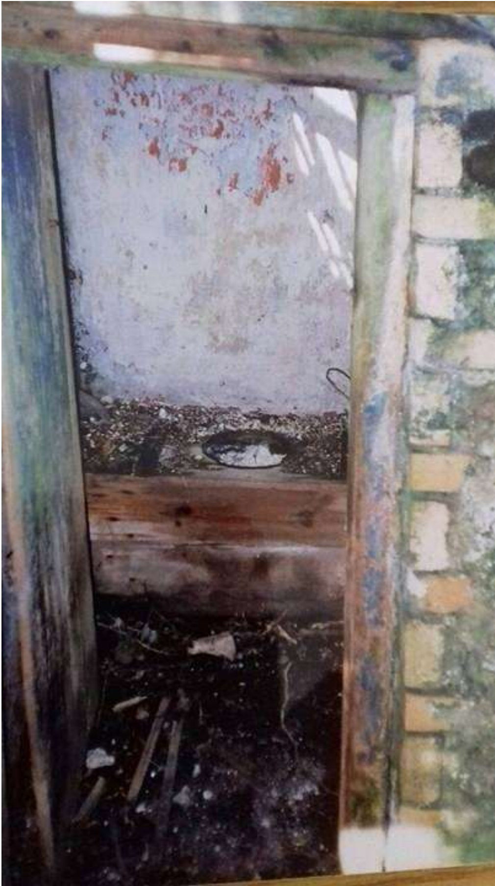
Figure 13: Victorian outside privy in need of TLC, pictured in the late 1990s before the house was renovated.
