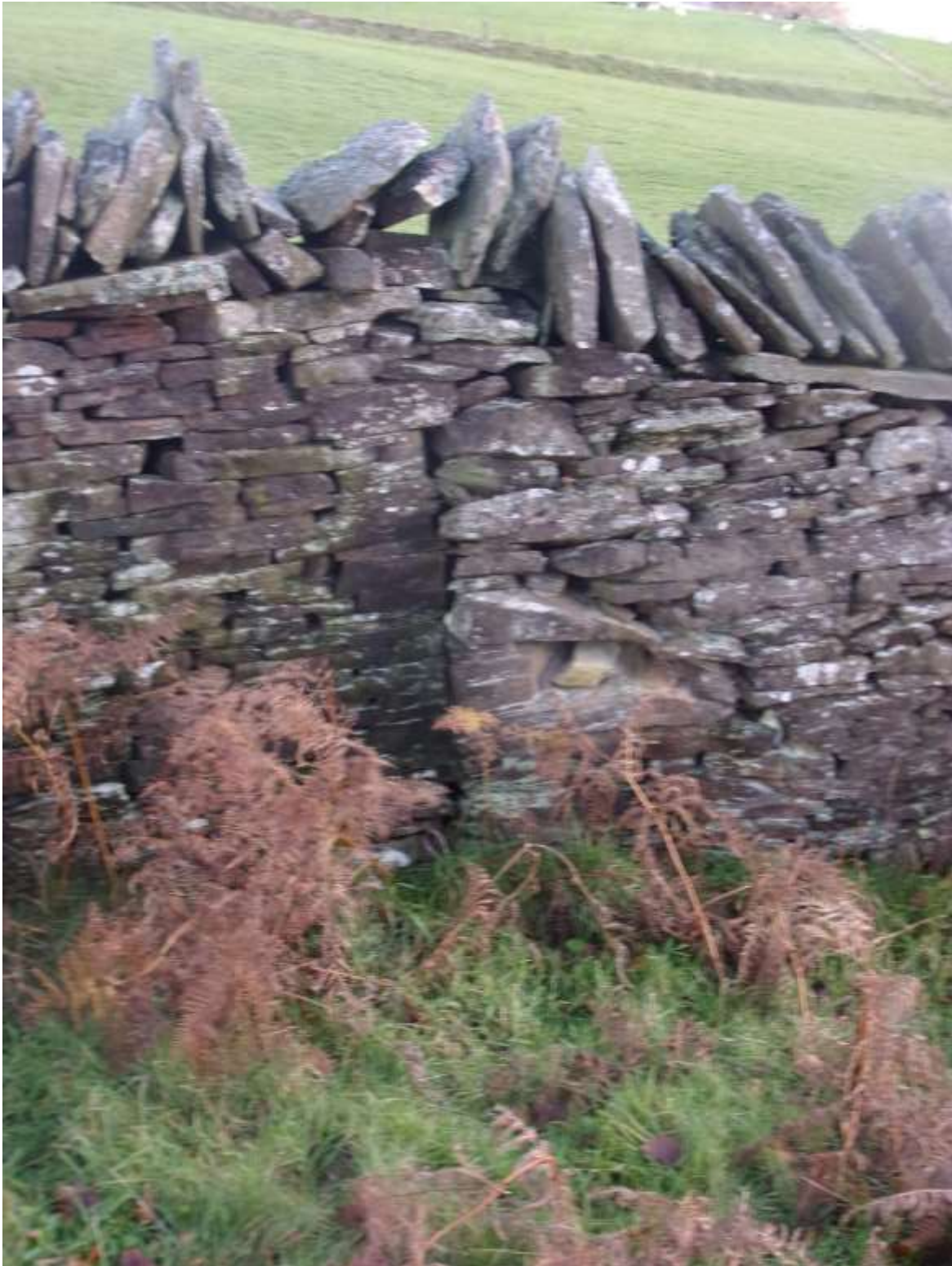
Figure 7 the lower remaining portion of original eastern gable wall has been badly tied into a dry stone wall of inferior construction (© R J Southall)
