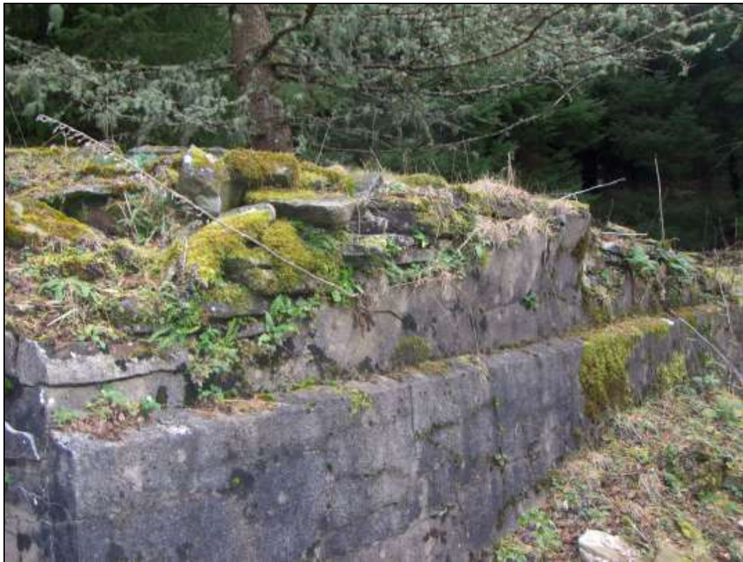
The lower pediment of the cow house which was strengthened with concrete in the 1920s.
